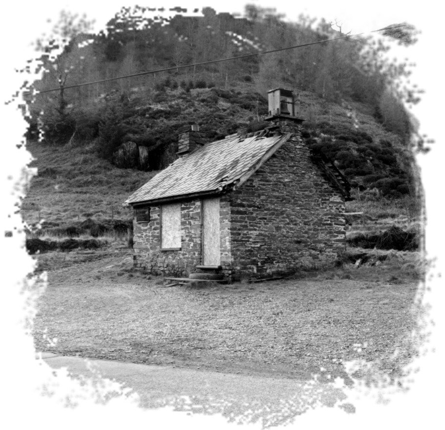
Below left is a rear view of the building, taken In 2002, showing the advanced state of dereliction.
